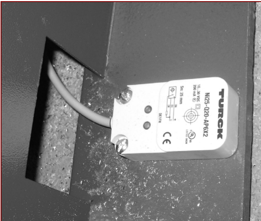
Figure 51 – Location of Lower Limit Switch, Control Cabinet, Reference Only
