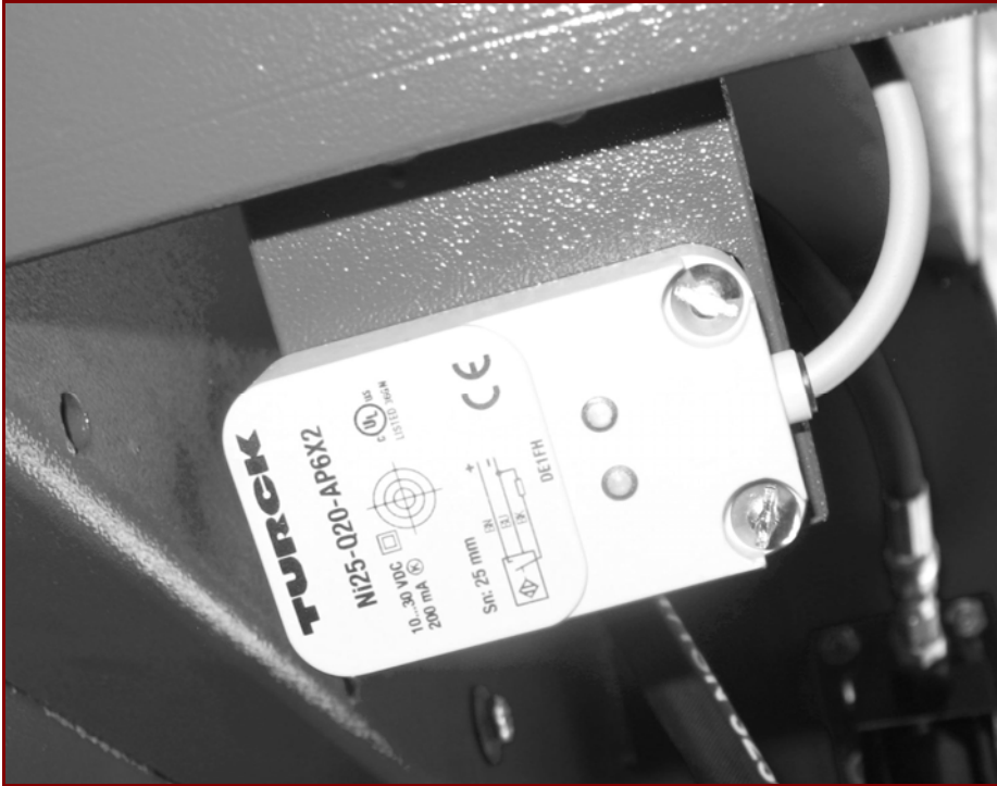
Figure 50 – Location of Upper Limit Switch, Control Cabinet
